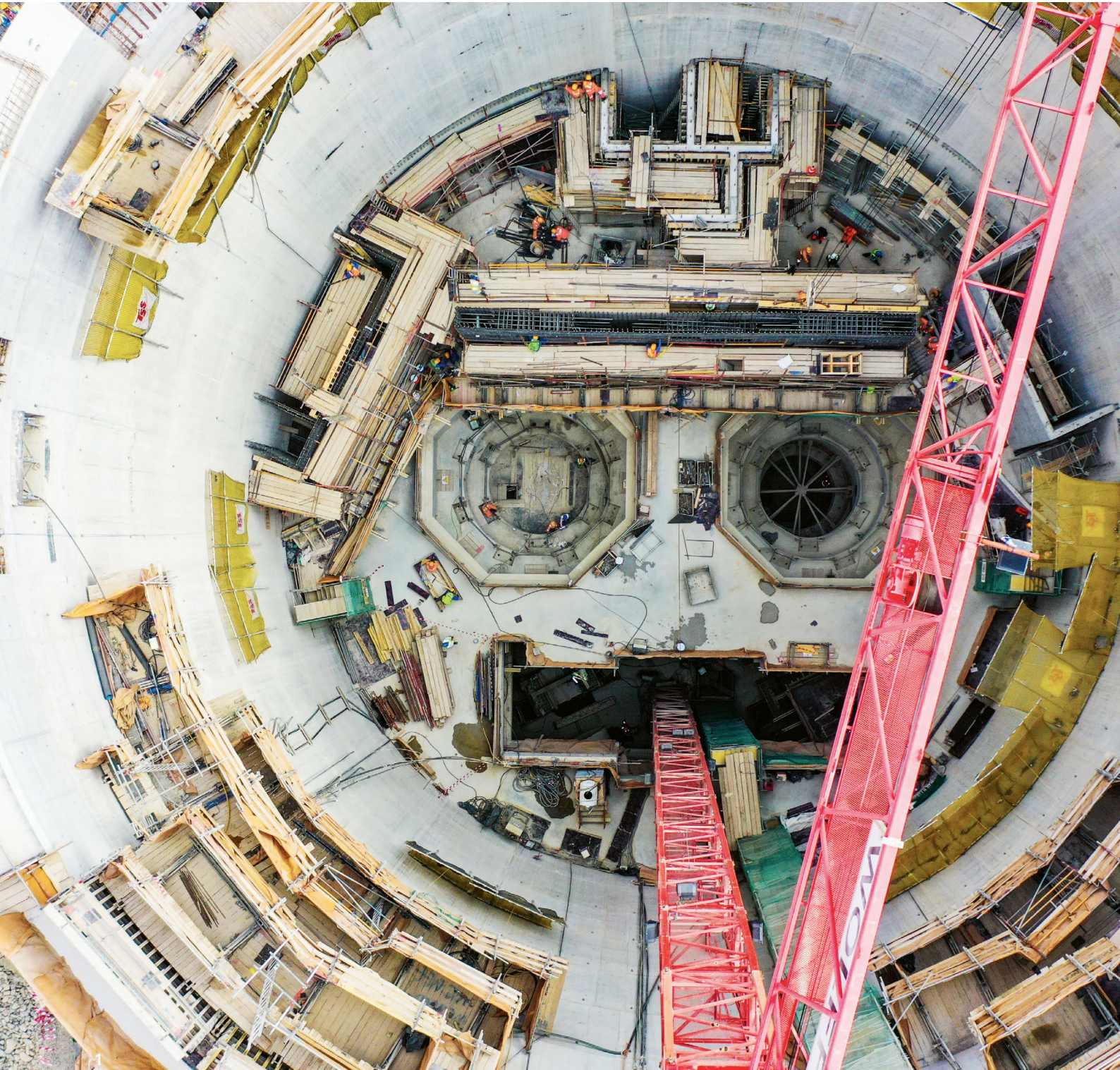
1 Hatta Pumped Storage Hydro Power Plant, Dubai, UAE
